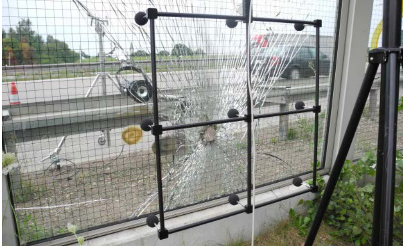
Figure 9: test setup for measurement of transmission loss of noise barrier with defect in situ
