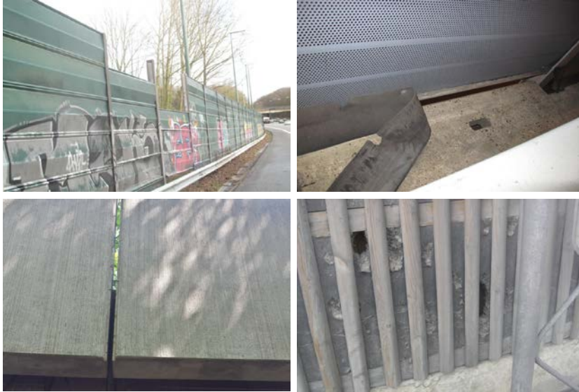
Figure 3: diverse defects at noise barriers; from top left to bottom right: absent aluminum element of noise barrier, leakage in the shape of a slit due to absent ground sealing, slit due to absent sealing between concrete elements of noise barrier, holes in insulating material of a wooden noise barrier due to mechanical impact (sources: BMVI; Walloon Road Administration, Belgium)
